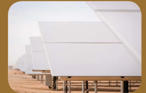
The Sheikh Zayed Solar Power Plant in Mauritania, funded by MASDAR, will reduce emissions by approximately 21,225 tonnes of carbon dioxide annually. (Source: MASDAR)
