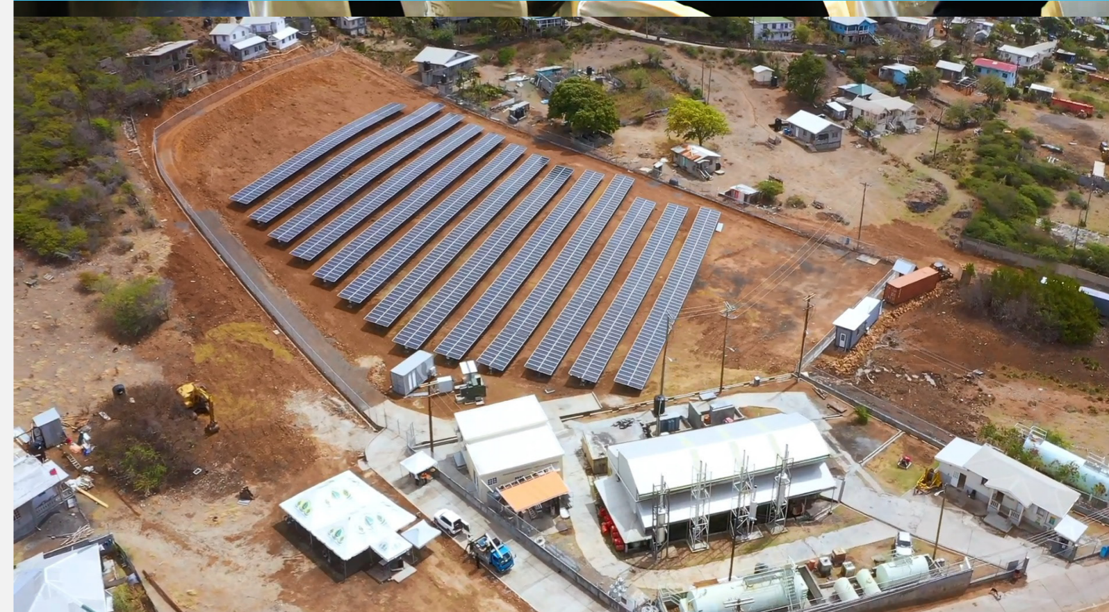
A 600 kW solar photovoltaic power plant in Saint Vincent and the Grenadines, equipped with a 637 kWh lithium-ion battery system. Source: MASDAR
